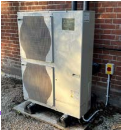
Newnham College Air Source Heat Pump
